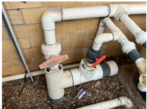
Photo #60 View of Small Pool return piping manifold.
