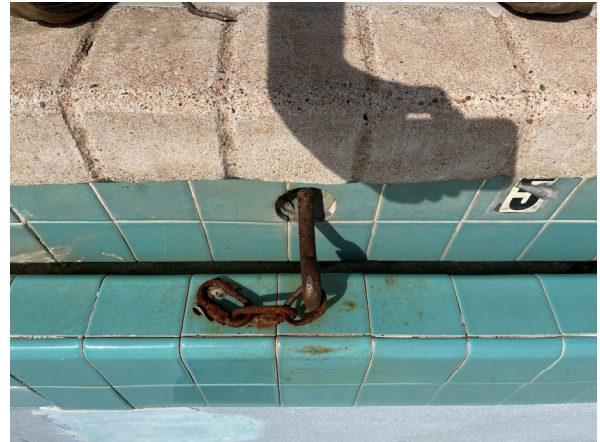
Photo #14 View of a Lap Pool wall anchor and rusted chain that appears to no longer be in use.
