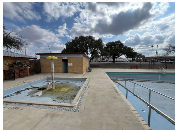
Photo #12 View of the pool deck that spans the gap between the Lap Pool and the Small Pool.
