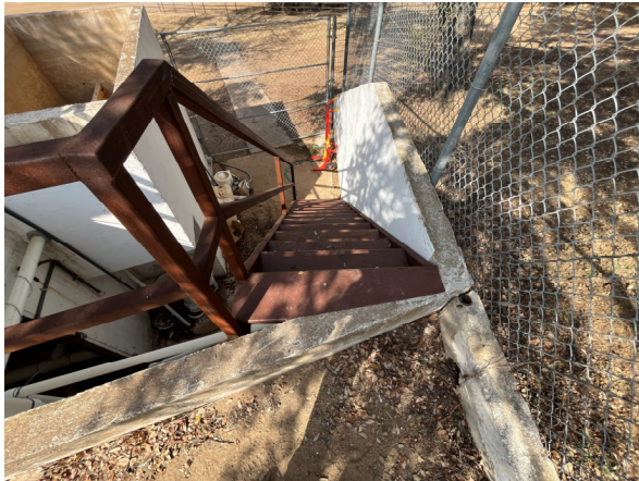
Photo #37 View of corroded stairs leading down to the main mechanical space.
