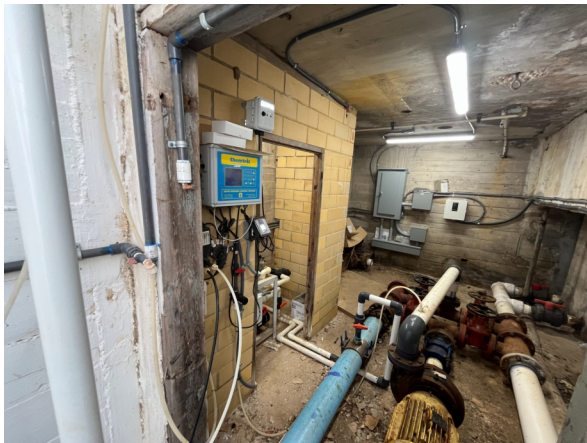
Photo #39 View of Lap Pool water chemistry controller and chlorine feed room.
