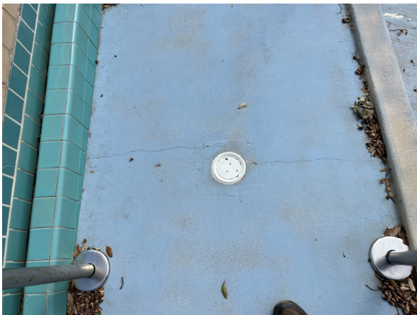
Photo #17 Example view of Lap Pool floor inlet serving the ramp entry.
