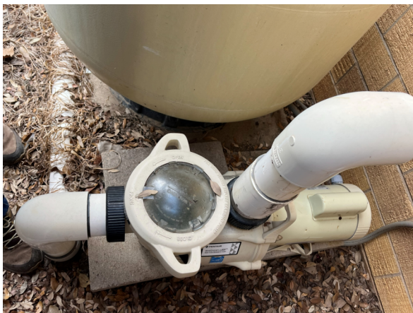
Photo #59 View of Small Pool recirculation/feature pump.
