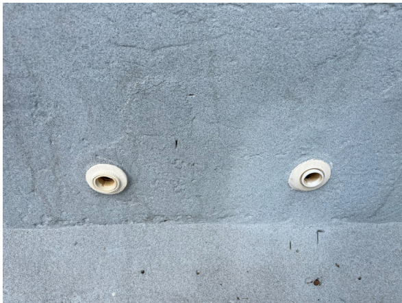
Photo #21 Example view of Lap Pool wall inlets – installed in sets of two (2).
