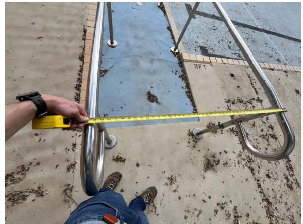
Photo #8 View of the 44" wide railings serving the ramp into the Lap Pool.
