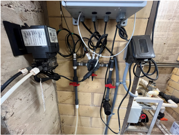
Photo #45 View of the water chemistry controller probes and muriatic acid feed pump.
