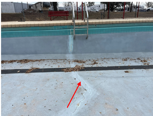
Photo #23 View of large crack that runs across the Lap Pool floor and south wall.
