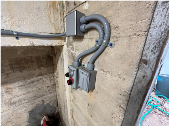
Photo #44 View of lighting control for the Lap Pool mechanical space
