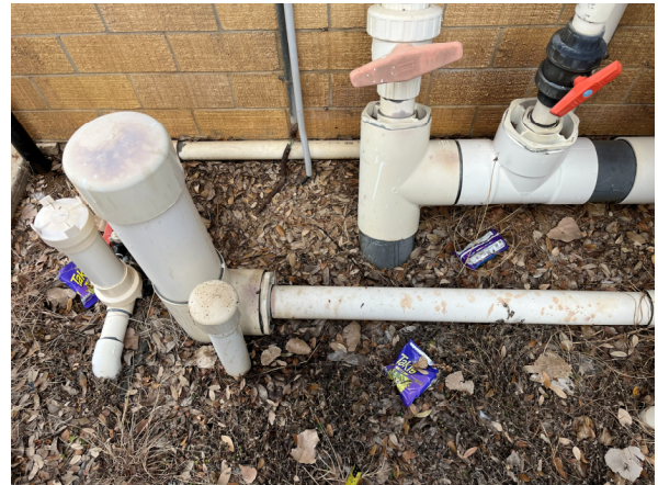
Photo #62 View of Small Pool return piping manifold.
