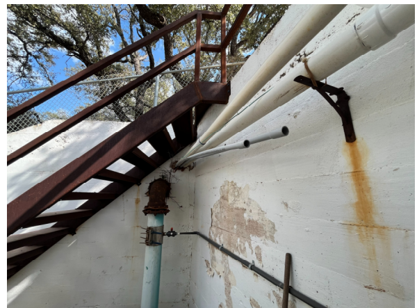
Photo #42 View of Lap Pool return piping.
