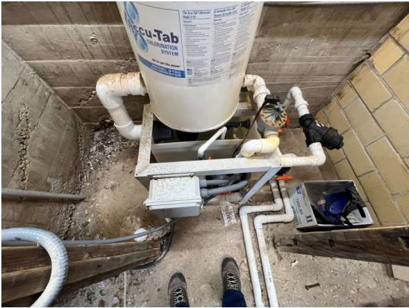
Photo #46 View of Lap Pool calcium-hypochlorite (solid chlorine) feed system.
