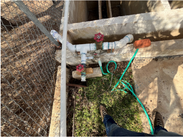
Photo #36 View of Lap Pool fresh water feed line.
