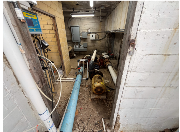
Photo #38 View of Lap Pool mechanical room.
