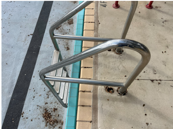
Photo #9 Example view of grab rails installed around the Lap Pool.
