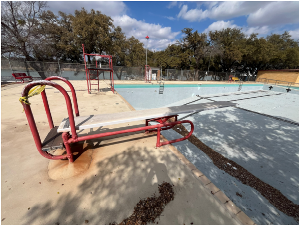
Photo #31 View of the broken diving board installed on the west side of the Lap Pool.
