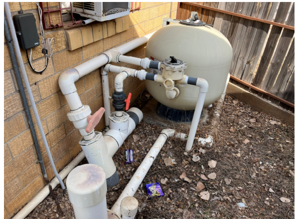
Photo #58 Example Small Pool mechanical systems.
