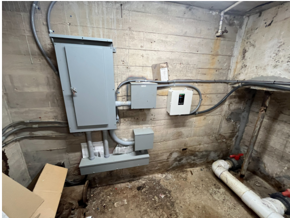
Photo #49 View of the Lap Pool electrical panels.
