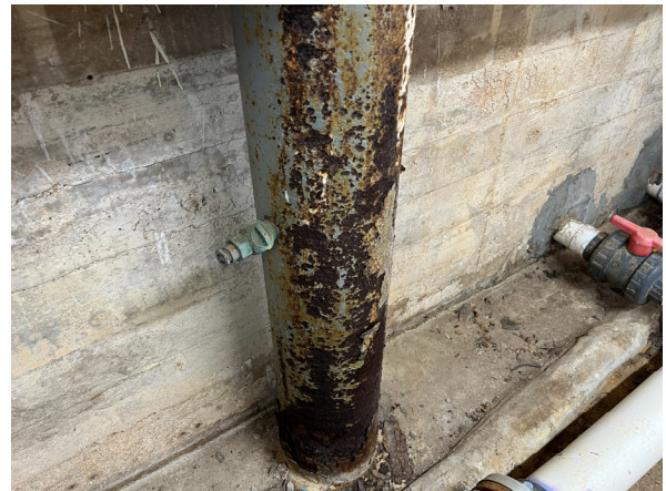
Photo #52 View of single equalizer line between Lap Pool main drains and surge weir.
